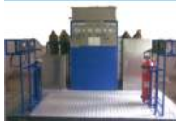
Helium Charging System
