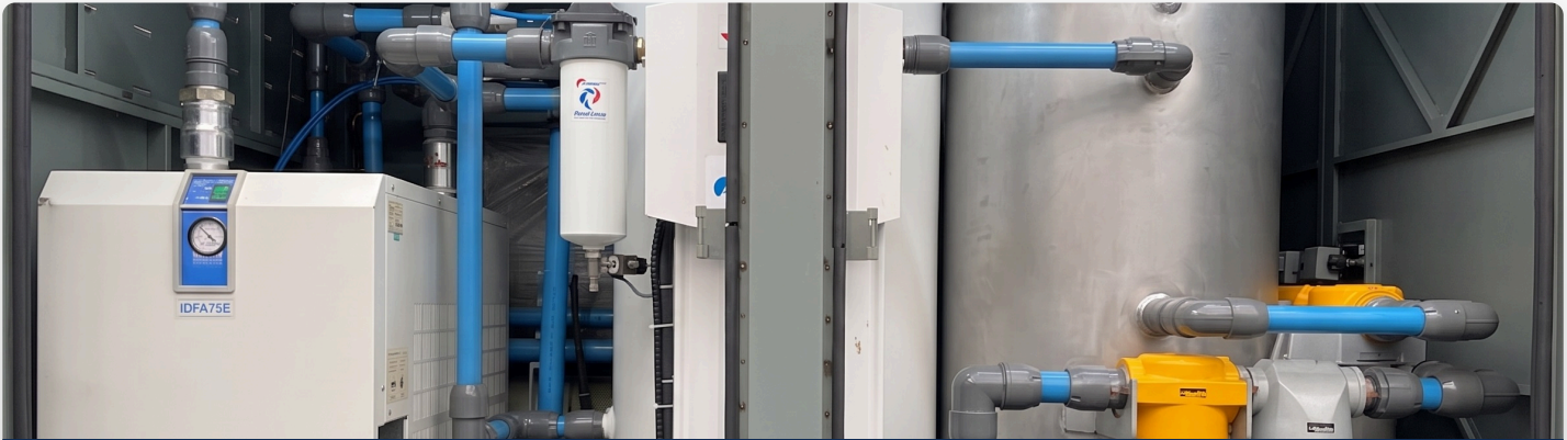
Nitrogen generation module interior — refrigeration dryer, PSA separation beds, buffer vessels and filter train
